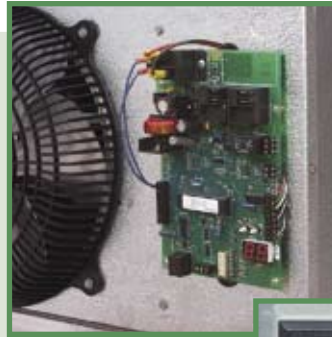
The Master Controller panel (shown above with housing removed) is mounted to the evaporator.
